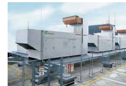
GPS3000 (M1T-03) for data center
