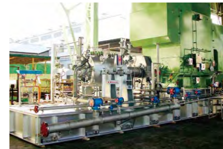
Motor-driven centrifugal compressor for pipeline (Saudi Arabia)
