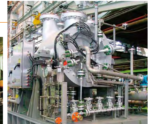
Gas turbine-driven centrifugal compressor for natural gas processing plant (Nigeria)
