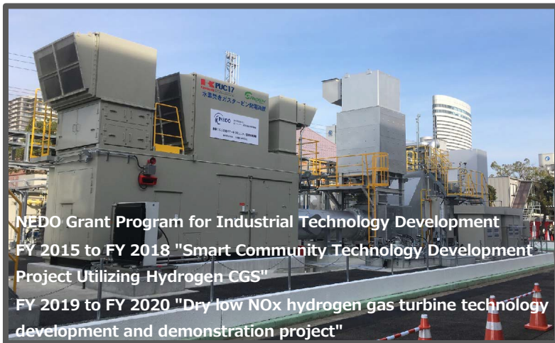
Hydrogen Gas Turbine Energy Center
