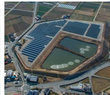
Figure 10: Kawasaki Trading Co., Ltd. Iwaoka Photovoltaic Power Generation Station: 1,505-kW power generation facility
