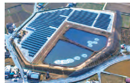
Kawasaki Trading Co., Ltd. Iwaoka Photovoltaic Power Generation Station: 1,505-kW power generation facility
