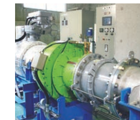
Micro hydropower system—generates electricity using a low flow water supply, such as a stream or agricultural waterway
