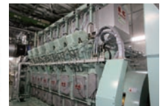
Kawasaki Green Gas Engine at Kobe Power Center
