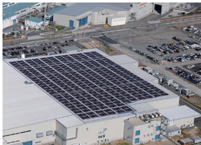
Photovoltaic power generation equipment with 750kW output installed at Nagoya Works 1
