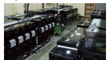
Battery power system for railways (New York subway verification test)
