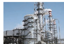
Flue gas Desulfurization System (Saudi Arabia)
