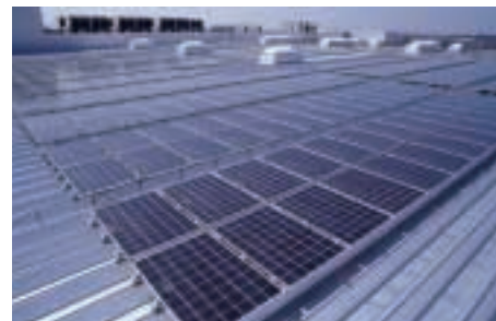
Photovoltaic systems at the Kawasaki Precision Machinery main plant (core parts plant)
