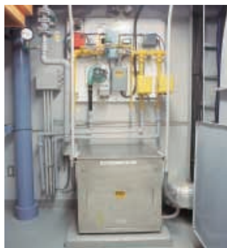
Burner control equipment
