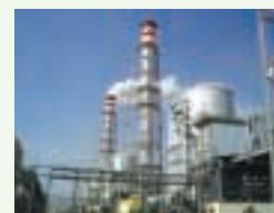
Flue gas De-SO x system (Saudi Arabia)
