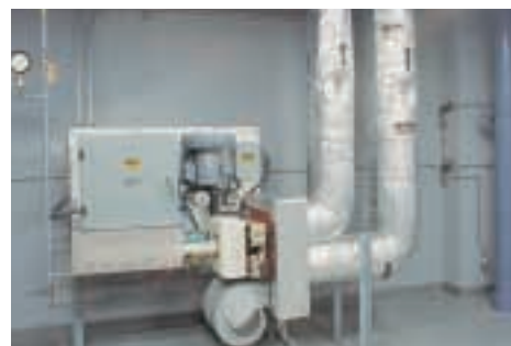
Mock smoke generation equipment
