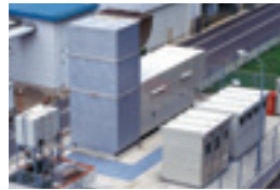
Emergency gas turbine generator
