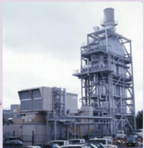
Combined cycle power plant (25 MW) equipped with Kawasaki gas turbine L20A
