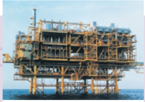
Gas compression module installed offshore
