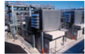
Gas turbine cogeneration system
