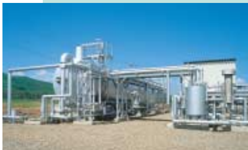
Biogas power generation plant in Yubetsu-cho
