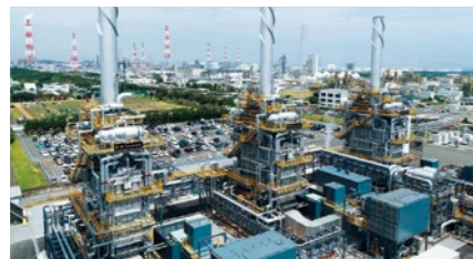
100 MW-class combined cycle power plant developed by Kawasaki
