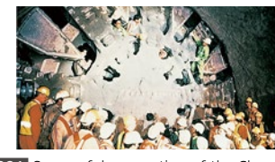
1991 Successful excavation of the Channel Tunnel, linking France and the United Kingdom
