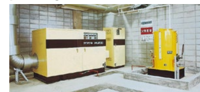
1976 Developed the Kawasaki GPS200 , the first Japan-made gas turbine generator
