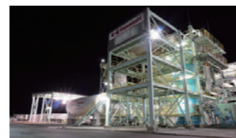
Hydrogen liquefier used for demonstration operation
