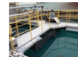
Wastewater treatment facilities
