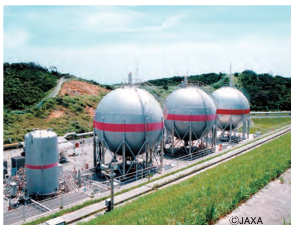
Fig.4 Japan's largest LH 2 tank
