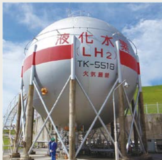
Hydrogen storage tanks
