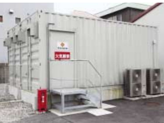
A container outfitted with an electric power supply-and-demand controller for research.
