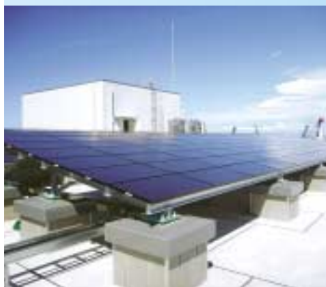
Photovoltaic power generation system.
