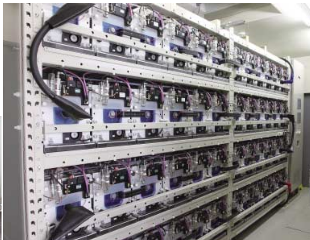
Inside the container, 48 GIGACELL modules are connected in series and record important data.
