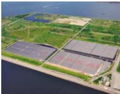
Sakai Solar Power Plant, connected to the Ishizugawa Substation (photo courtesy of KEPCO).
