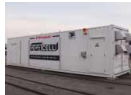
The system stored in a 40 ft. container
