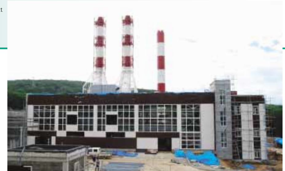
Exterior of the district heating power plant (Marine Center Site) in September.
