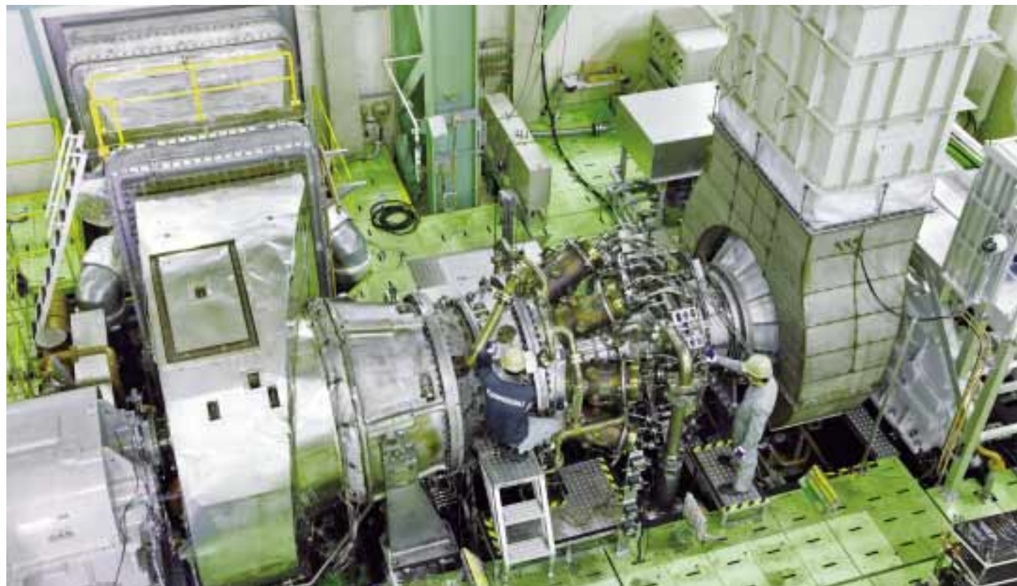
Kawasaki's 30 MW class L30A Green Gas Turbine undergoing trial runs at the Akashi Works. A cogeneration system built around the L30A has a combined thermal efficiency of over 83% and NOx emissions are cut to the world's lowest level.
