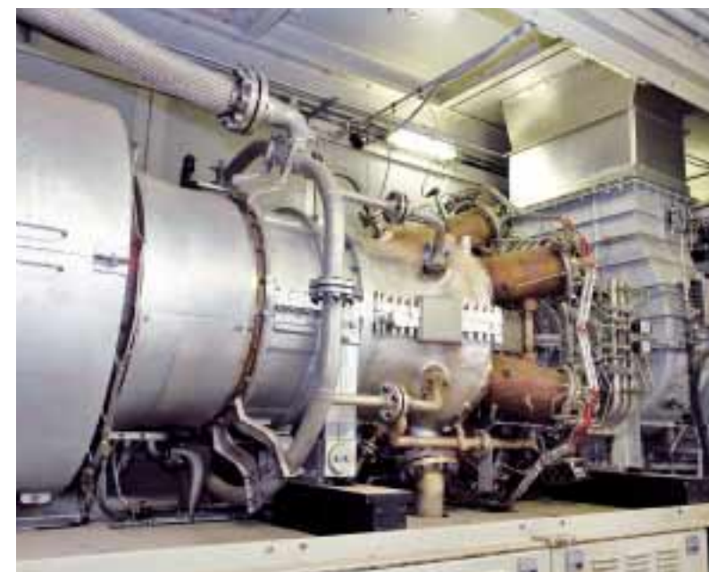
The five generators come equipped with Kawasaki's M7A-02D Green Gas Turbine.
