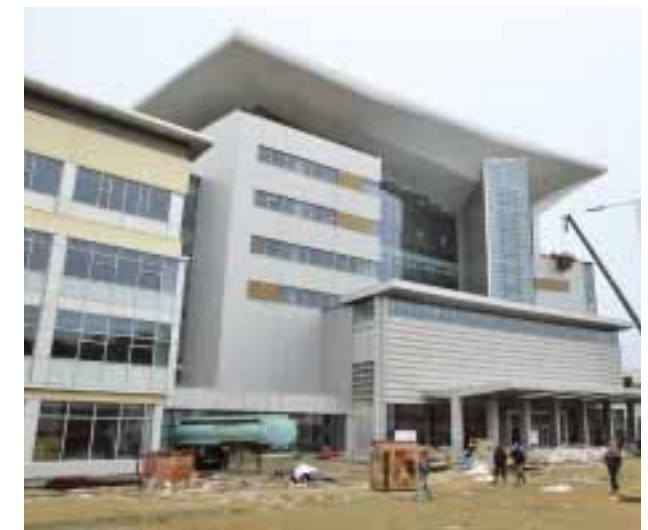
The Main venue of the APEC summit, where the summit was held, under construction.
