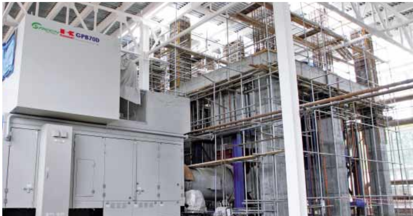
Inside the building. Two Kawasaki Green Gas Turbine generators (GPB70D) are installed, waiting to begin trial operation.
