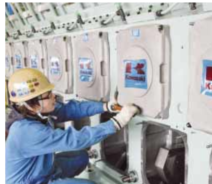
Work proceeds on schedule at the assembly plant. Kawasaki raised the production capacity of Kobe Works to four engines a month, to meet the growing demand both at home and abroad.
