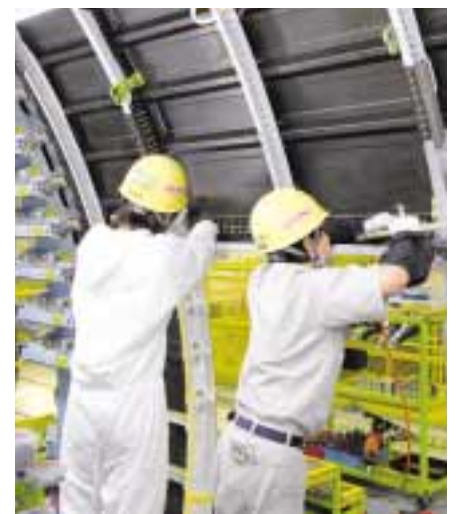
▶ The forward fuselage is turned clockwise as its internal structure is assembled to boost work efficiency. Kawasaki earned high marks from Boeing for outstanding productivity.
