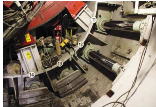
Whenever 1.1 m of soil is excavated, the shield jacks are retracted and segment blocks laid in.
