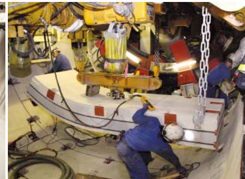
An erector lifts a segment block and moves it into place for installation. Workers must stay on their toes in the cramped environment.
