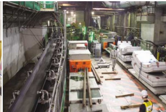
The underground shaft area where construction work began. Soil is carried out via conveyor belt while segment blocks are loaded on a tram.
