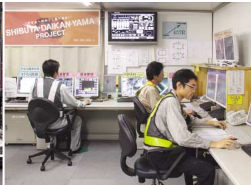
The central control room 20 m below ground is the project's nerve center.
