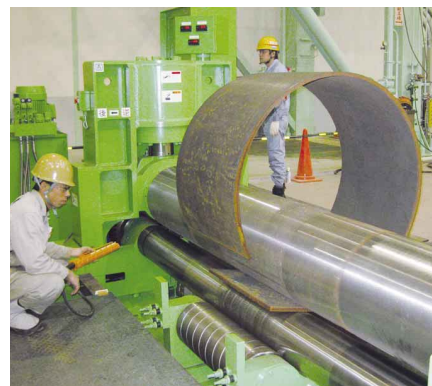
▶ A pressing machine bends the steel plate to form a cylinder (tube).
