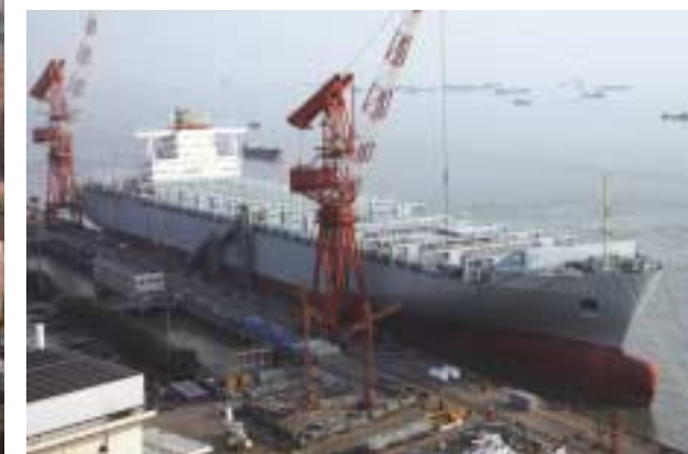
Outfitting quay to be expanded from 540 m to 920 m in the second expansion phase.
