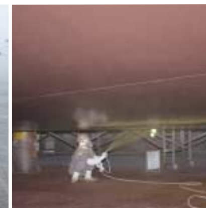
Coating a ship with paint. The coating process, which prolongs the life of a ship, meets the new, stricter international standard.
