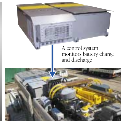
Major electric devices are mounted on the roof.
