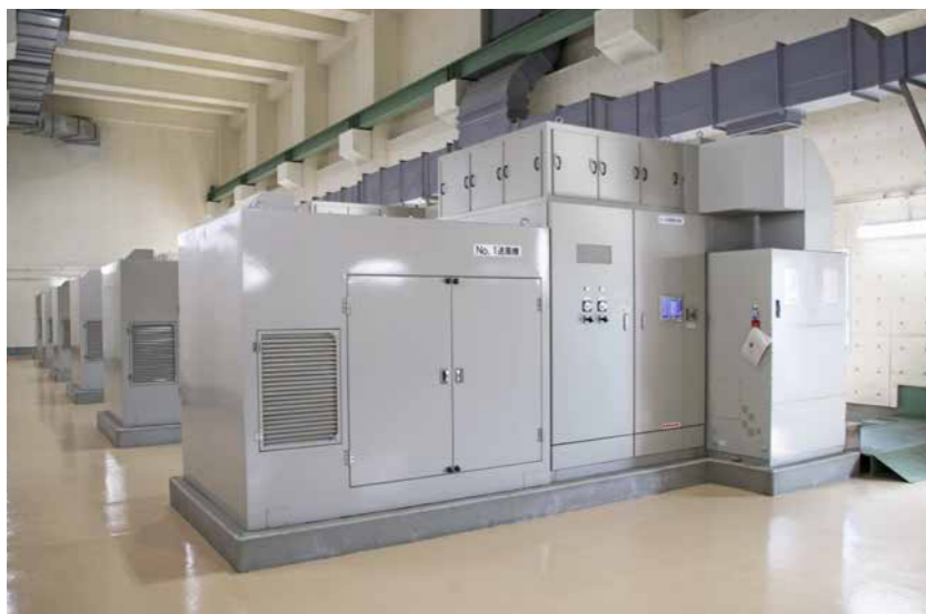
In the new blower/pump station building, six units of the MAG Turbo M25 are in operation.
