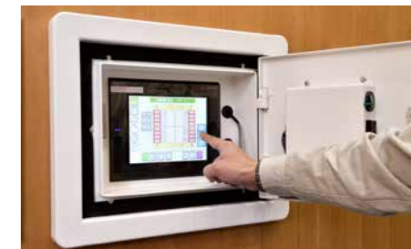
The control panel for the floor conversion system. If someone enters the arena while the conversion is taking place, the system activates a safety mechanism to stop the operation automatically.
