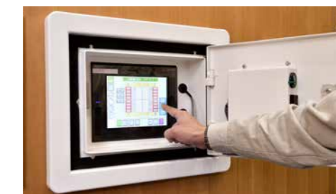
The control panel for the floor conversion system. If someone enters the arena while the conversion is taking place, the system activates a safety mechanism to stop the operation automatically.
