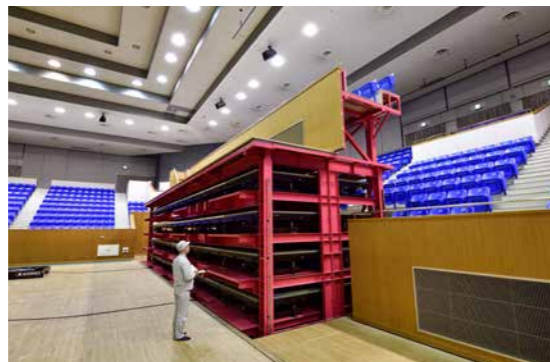
These storage lifters are located under the front row of seats and the area of the arena immediately in front of the seats. During operations, they are raised and lowered to unload/reload the tatami units and AGVs.
